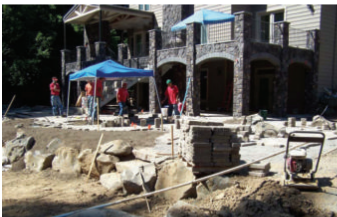
The crew set the pavers on top of a 6-inch compacted gravel base with a 1-inch sand topping.
